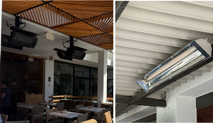
Mounted electrical heaters
