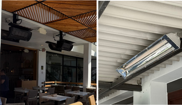
Mounted electrical heaters
