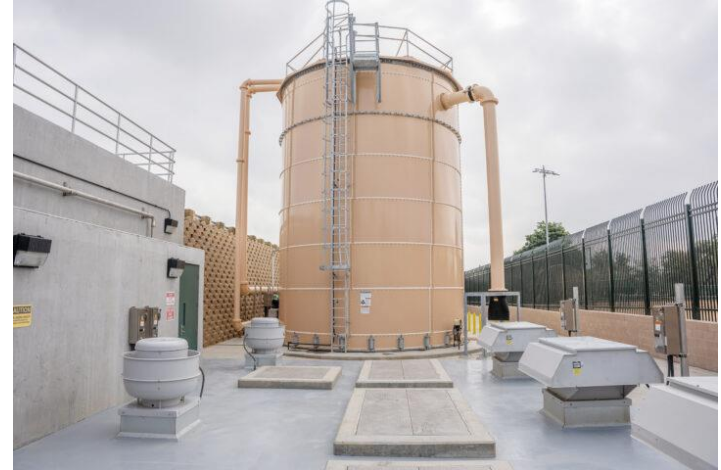
Peck Iron and Manganese Treatment Plant (Local Wells)
