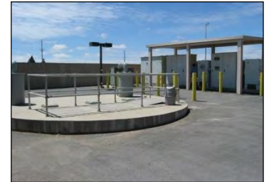
Camarillo Pump Station No. 2
