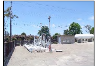
Reservoir No. 1 Pump Station
