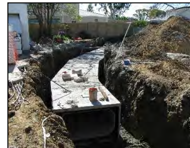
Flomar Storm Drain
