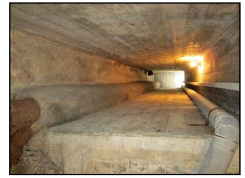
Sewer Lift Station No. 3
