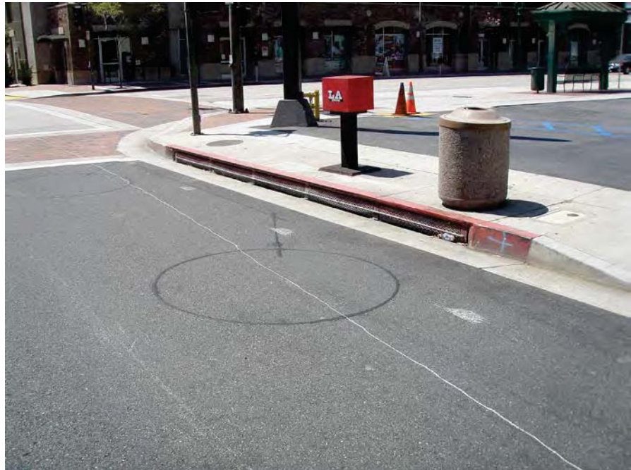
Curb inlet grate catching debris (Credit: Andre Haghverdian)
