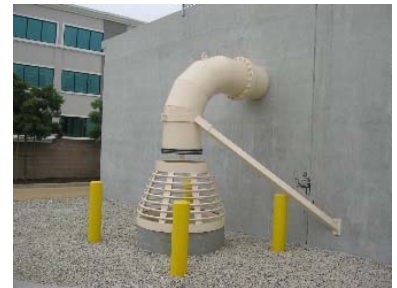
Reservoir Overflow Airgap at St. Joseph Reservoir
