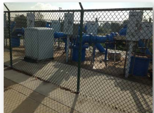
Existing On Site Booster Pump Station
