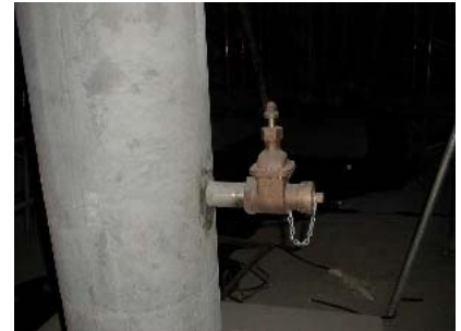
Reservoir Wash-down Piping
