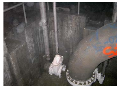
Drain Sump and Valve
