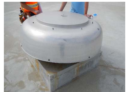
Reservoir Roof Vent with Exhaust Fan
