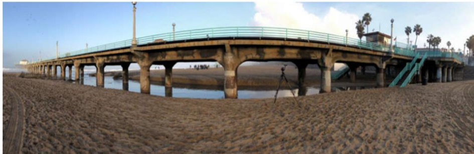
Figure 25: January 2019 King Tides, Beach Erosion
