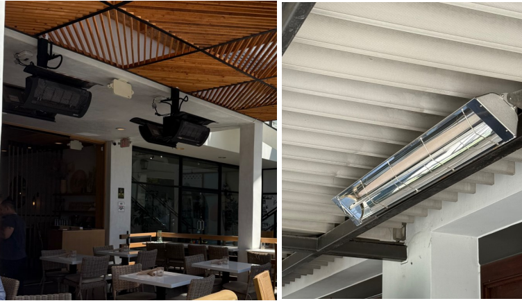
Mounted electrical heaters
