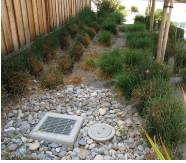
Figure 6.3233 Vegetated bioswale filters stormwater
